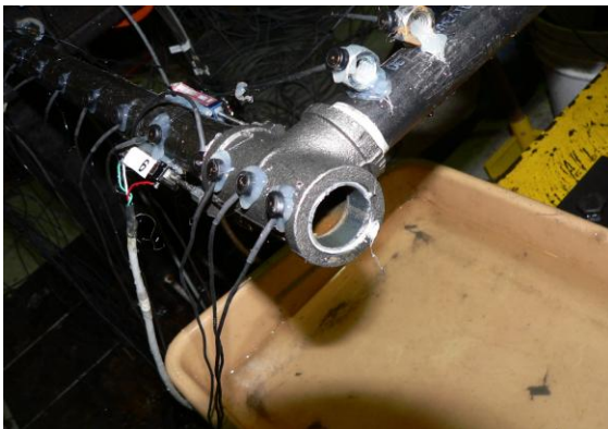
Pipe fractured at the edge of tee
