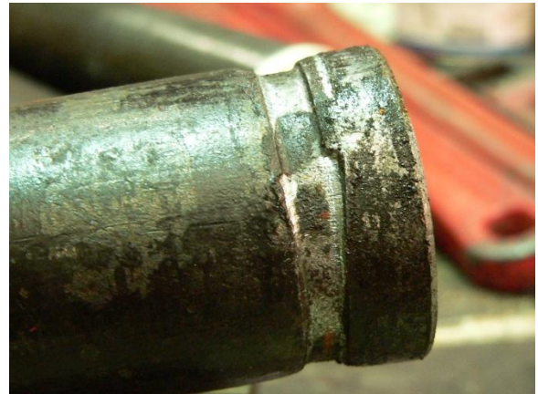
(f) Wearing damage around the groove in the pipe
