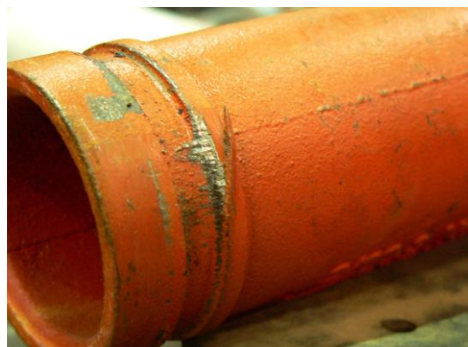
Groove of tee joint wore away
