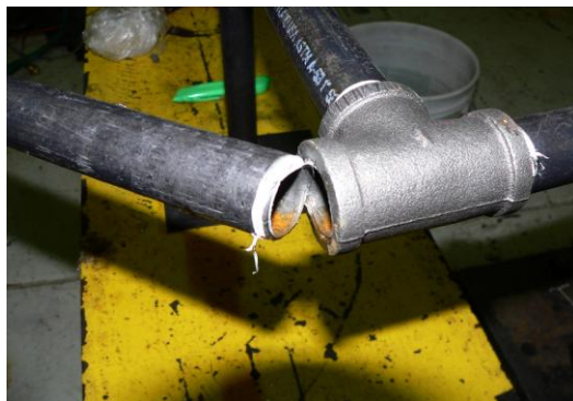
Pipe fractured at the edge of tee
