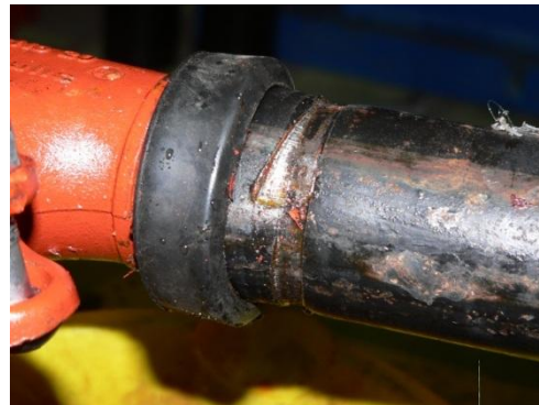
Groove of pipe wore away
