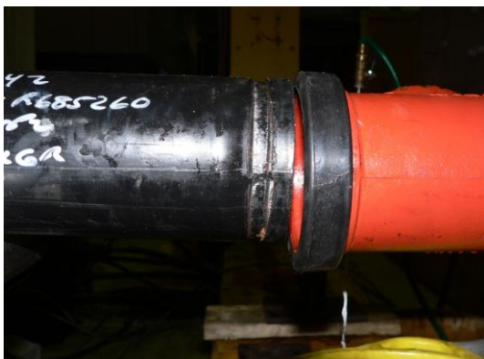
Groove of pipe wore away
