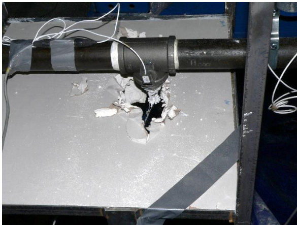
(a) Damage of rigid ceiling box (Configuration 1-6, 100% MCE level)
