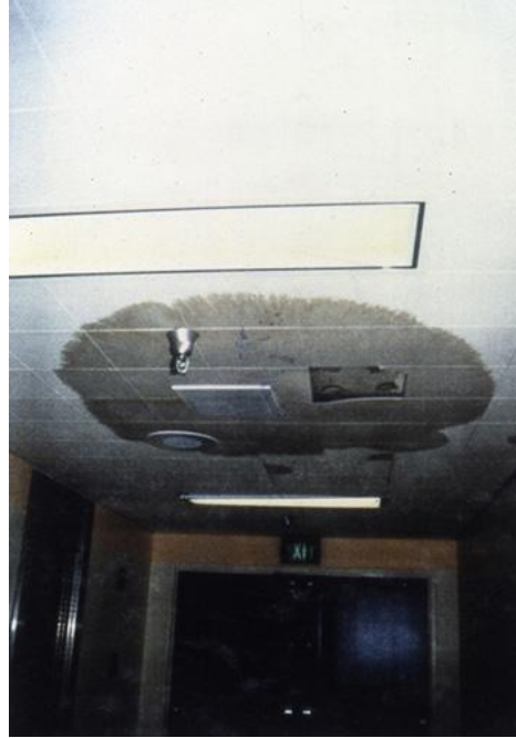
Figure 1-7 Water leakage caused by pipe damage at joint (from Degenkolb Engineers, 1994)
