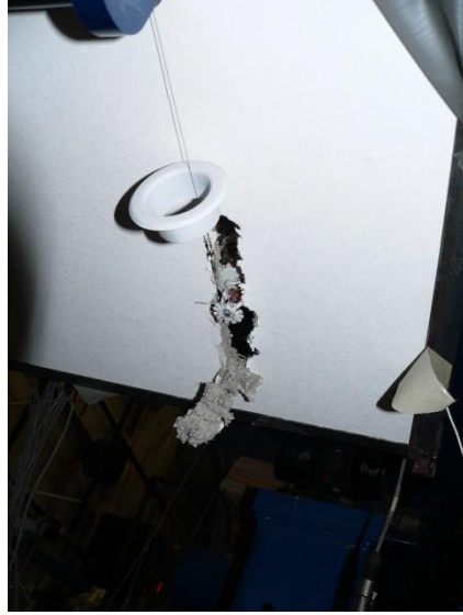
Figure 4-43 Damage of ceiling box
