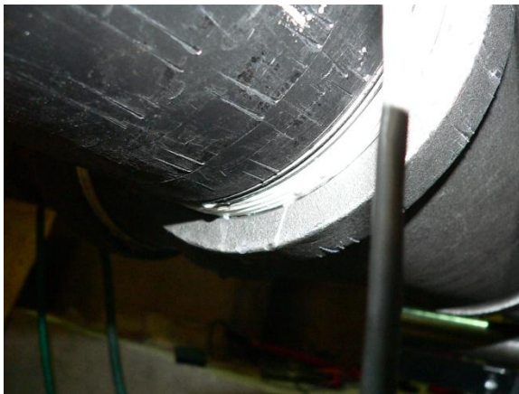
Gap generated between pipe and tee joint due to imposed bending
