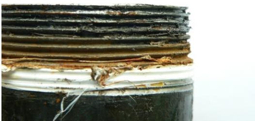
Pipe threads erode due to slippage
