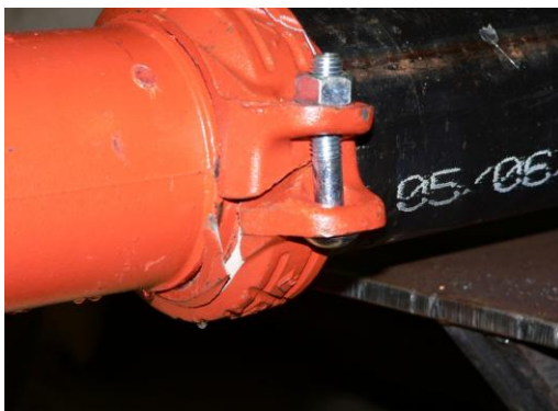
Coupling flange fractured
