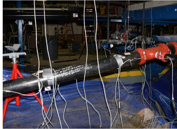
(b) Excessive deformation of main line after failure of vertical hanger (Configuration 3-5, 100% MCE level)
