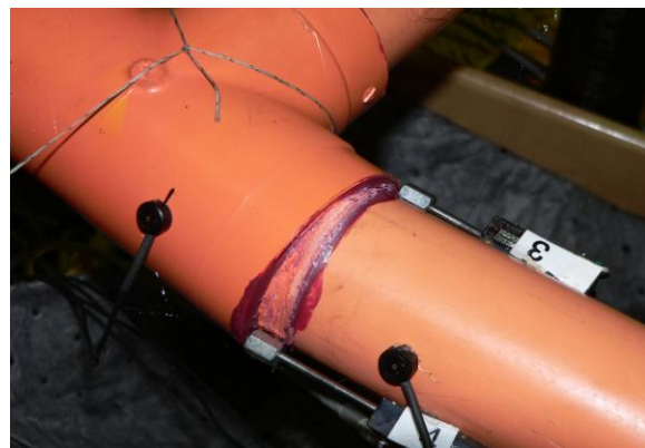
Cement Glue slipped
