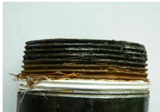
Thread sealant (Teflon tape) degraded
