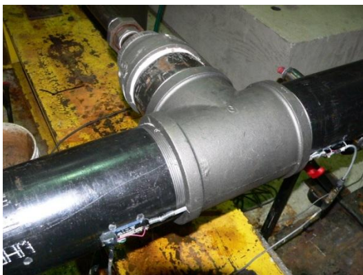
Pipe threads slip from tee threads
