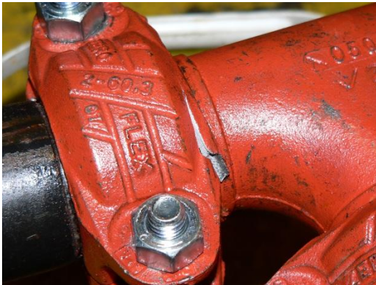
(a) Fracture of coupling flange initiated from the housing key
