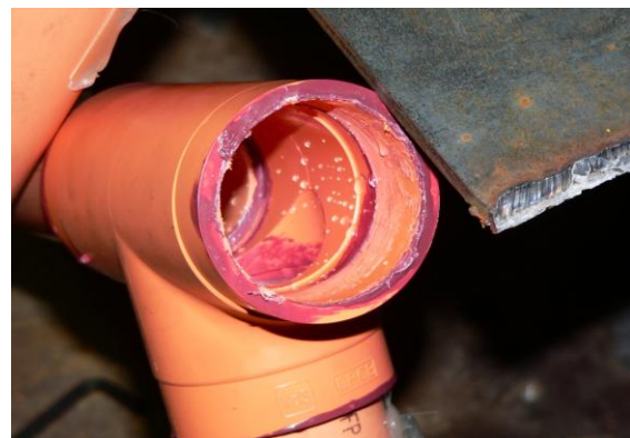
Pipe peeled off the inner surface of tee joint
