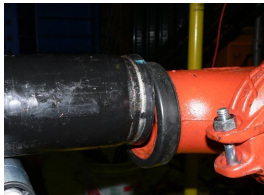
Groove of pipe wore away
