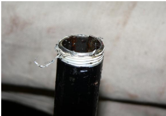
Pipe threads erode due to imposed rotation
