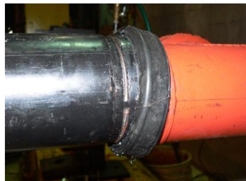
Groove of pipe wore away
