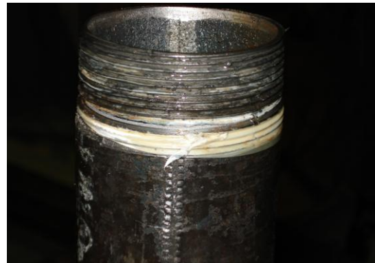
Thread sealant (Teflon tape) degraded
