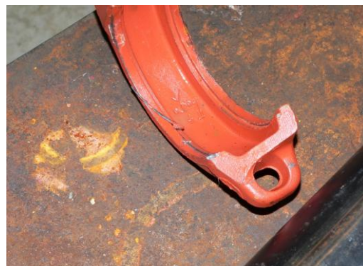
Coupling flange fractured
