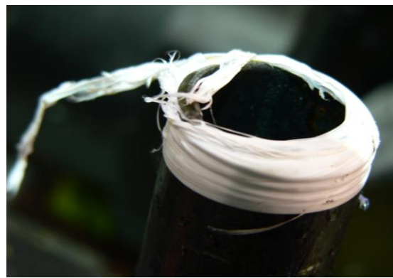
Thread sealant (Teflon tape) degraded
