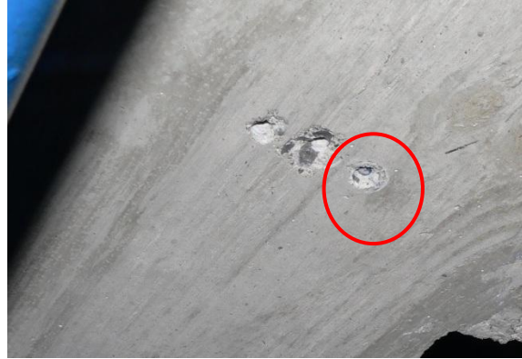
(b) Remnant of SAMMY screw in the concrete slab (Configuration 1-5, 100% MCE level)
