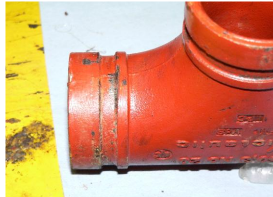
Groove of tee joint wore away
