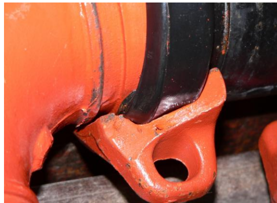
Groove of pipe wore away
