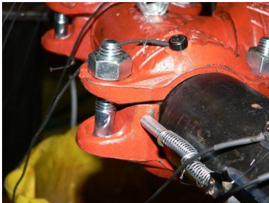
Gap generated between flange couplings
