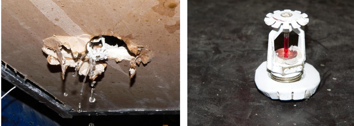
Figure 4-36 Failure of quick response pendant sprinkler head (Configuration I-6, 100% MCE level)
