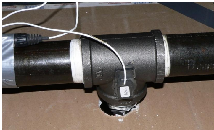
Figure 4-24 Accelerometer attached to the tee joint connected to sprinkler head
