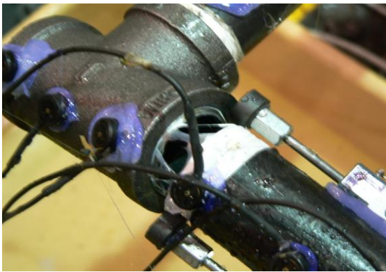
Pipe fractured at the edge of tee
