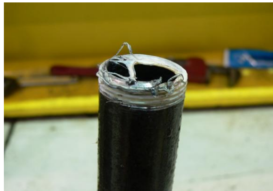
Thread sealant (Teflon tape) degraded
