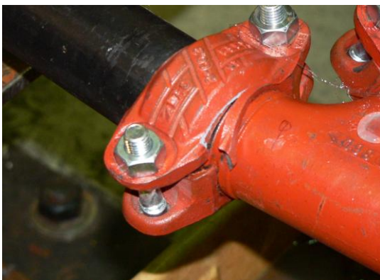
Coupling flange fractured
