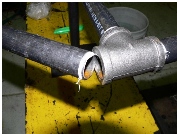
(e) Fracture of pipe
