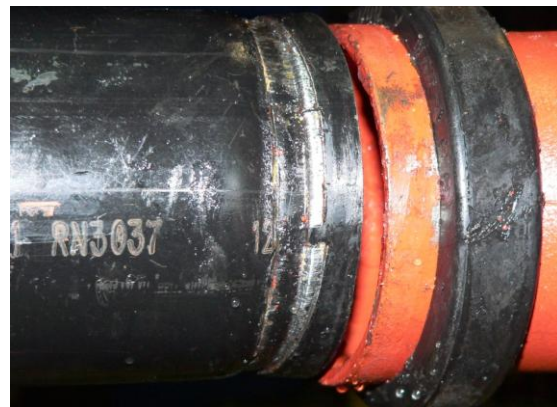
Groove of pipe wore away
