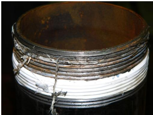
Thread sealant (Teflon tape) degraded
