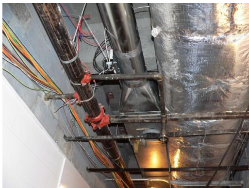
(e) Steel pipes with Groove-fit joints
