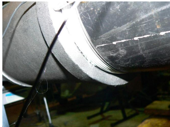
Thread sealant (Teflon tape) degraded
