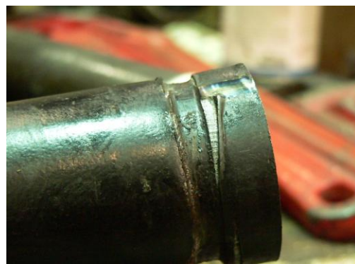
Groove of pipe wore away
