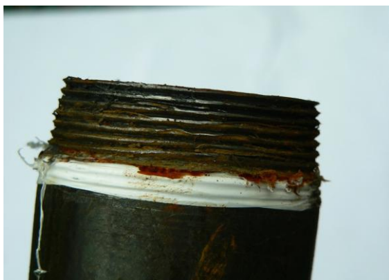
Pipe threads erode due to slippage
