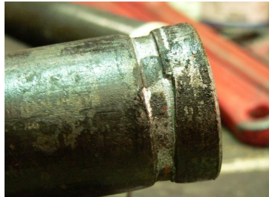
Groove of pipe wore away
