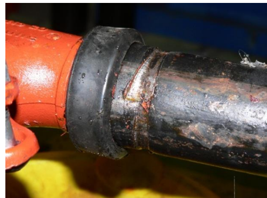
(d) Wearing damage around the groove in the pipe
