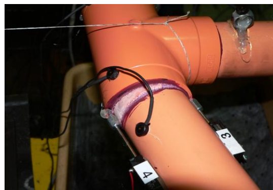
Cement Glue slipped
