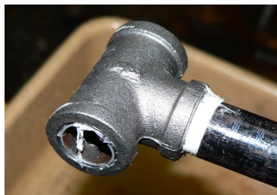
Pipe fractured at the edge of tee
