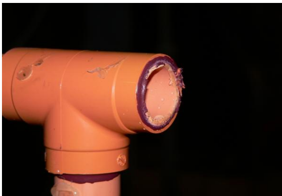
Pipe fractured at the edge of tee
