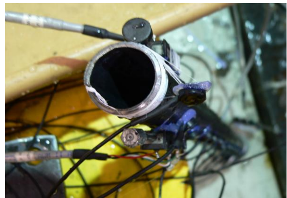
Thread sealant (Teflon tape) degraded
