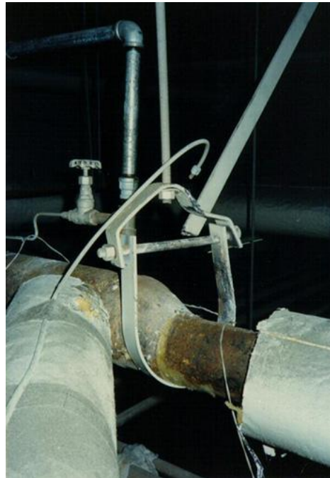
Figure 1-8 Failure of lateral bracing system (from Mason Industries, 1994)
