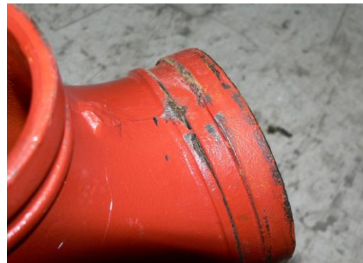
Groove of pipe wore away
