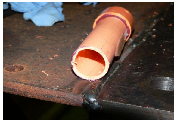
Pipe fractured at the edge of tee
