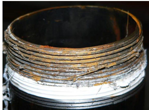
Thread sealant (Teflon tape) degraded
