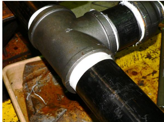
Gap generated between pipe and tee joint due to imposed bending
