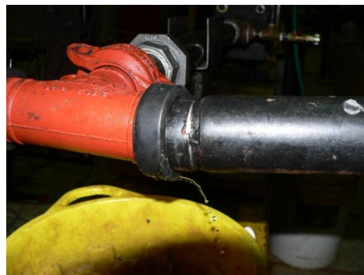
Groove of pipe wore away
