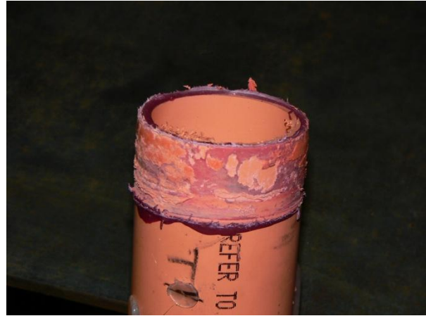
(b) Inner surface of the tee joints peeled off with the cement glue
