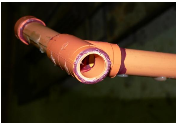
Pipe fractured at the edge of tee
