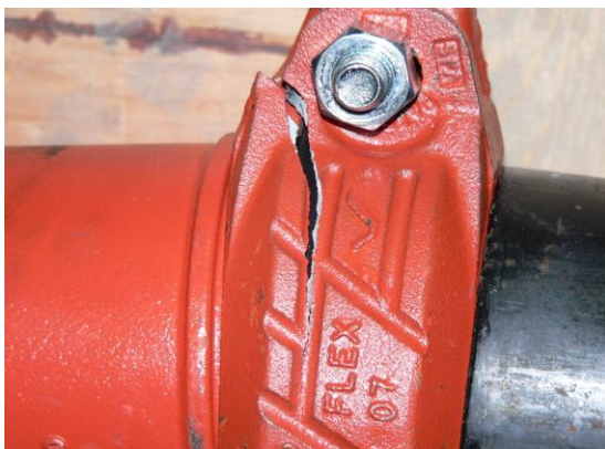
Coupling flange fractured
